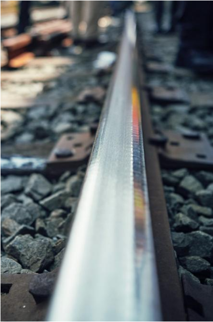
Fig. 4: The rail surface after only one pass - complete removal of the damage and exactly set target profile
