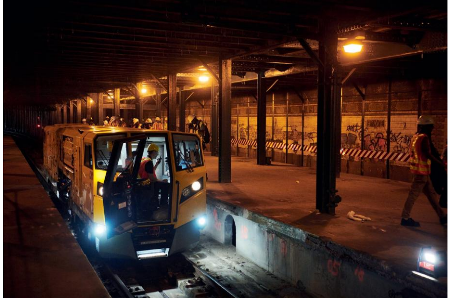
Fig. 5 The mobile high performance milling machine in use in a NYCTA station.
